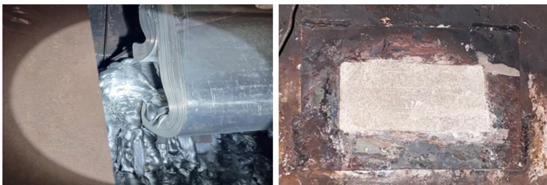
Figure 15. The location of metal tap-out from collector bar window showing the melted collector bar to cathode flexible connection (left), the same collector bar window after copper bar removal and sealed with refractory castable (right).
