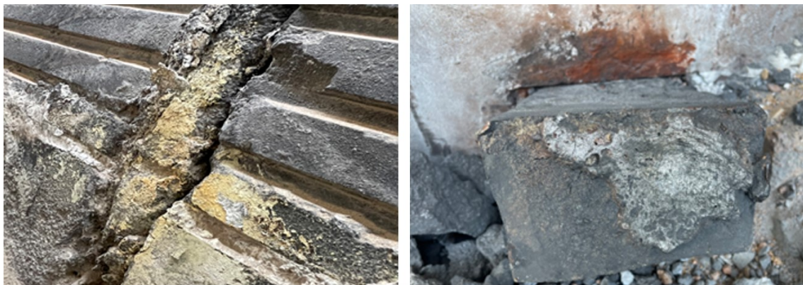
Figure 17. Al_4C_3 penetration through the T-joint and end face of cathode blocks (left), and cross-sectional cut of copper bar highlighting silver-colored Al-Cu alloy penetration just before entry into the cathode block (right).
